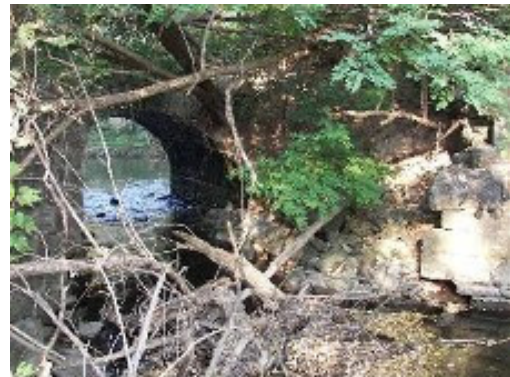
The trail has been closed due to the deterioration of this stone culvert, near Fishers Road.
